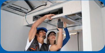
Air Conditioning System Design, Supply & Installation
