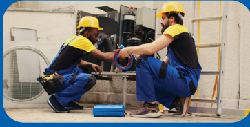
Annual Maintenance Contracts
